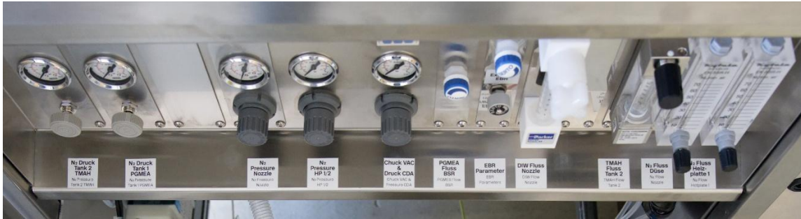
Figure 4: Flowmeters and regulators panel
